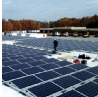
500 kW commercial system
